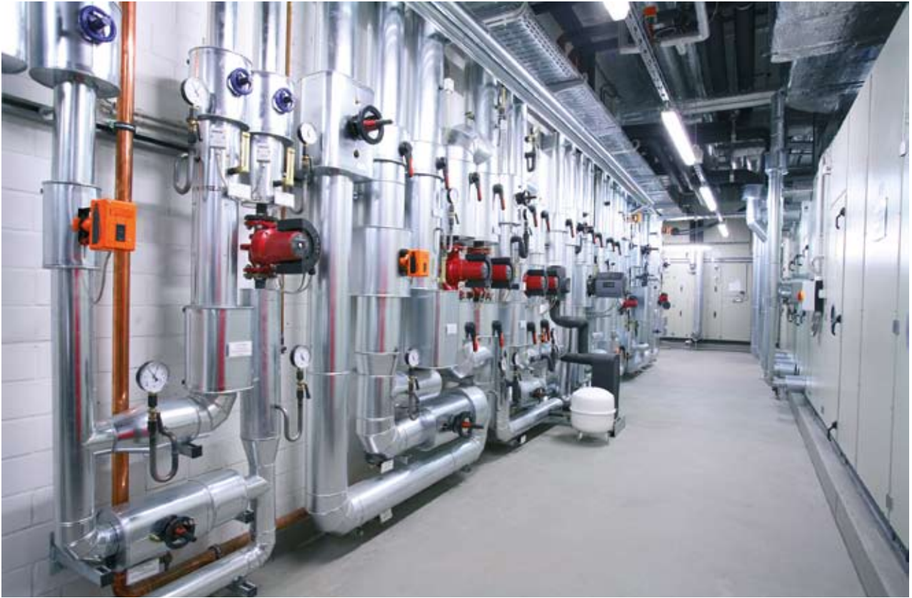
HVAC installation with MAGNA and E-pumps
